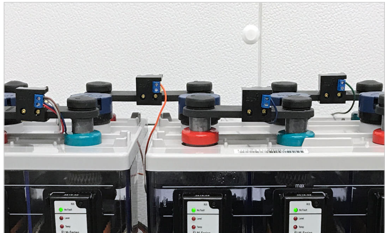
BQMS Battery Connection - C-Type Clamps
